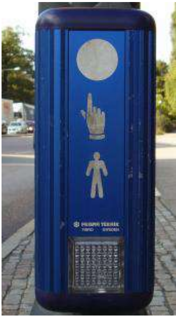
Traffic signal control at crossing.
